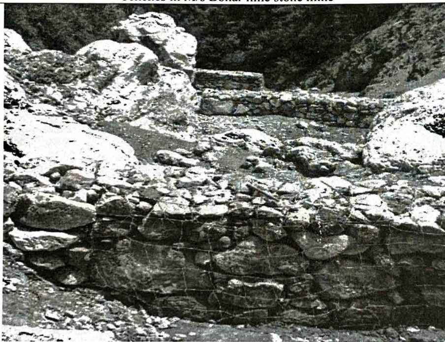
Photograph no. 6 – Shows status of retaining structures provided by M/s Bohar lime stone in the run off channel of seasonal dunga nallah to protect flow of debris and damage to property of local people
